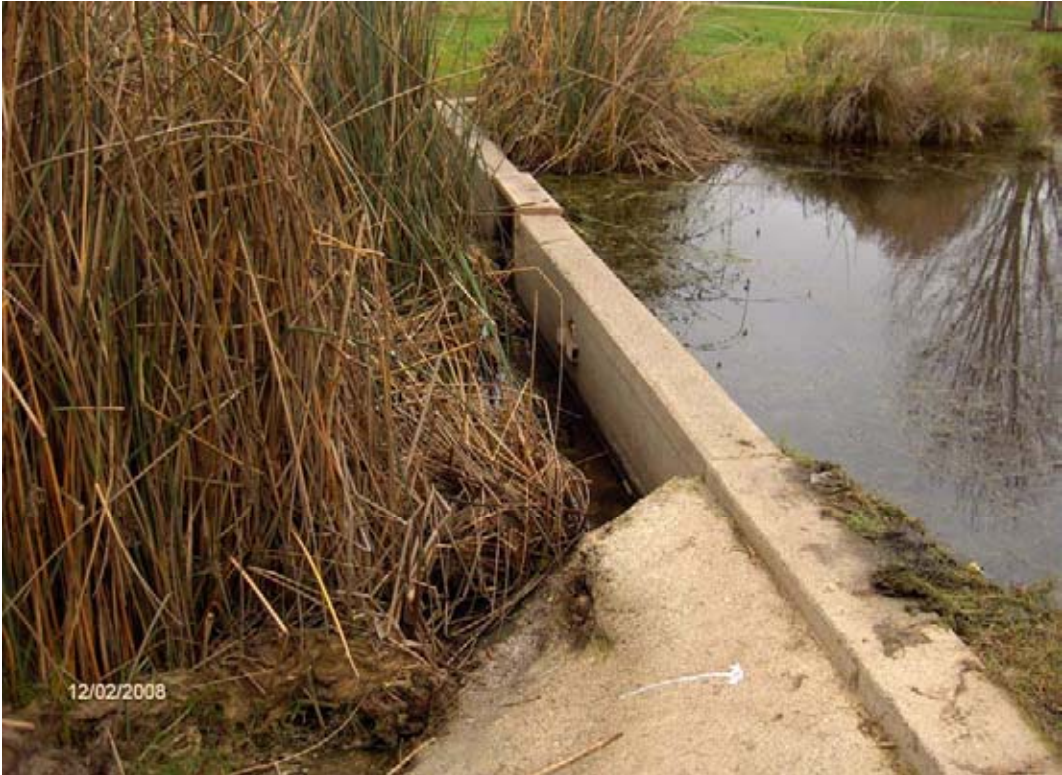
Photo of Camden Weir looking north. Pond on right side of photo. Downstream on left side.
